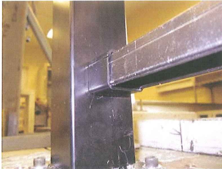
Photo No. 7 Bottom Rail Bracket-to-Rail Connection
