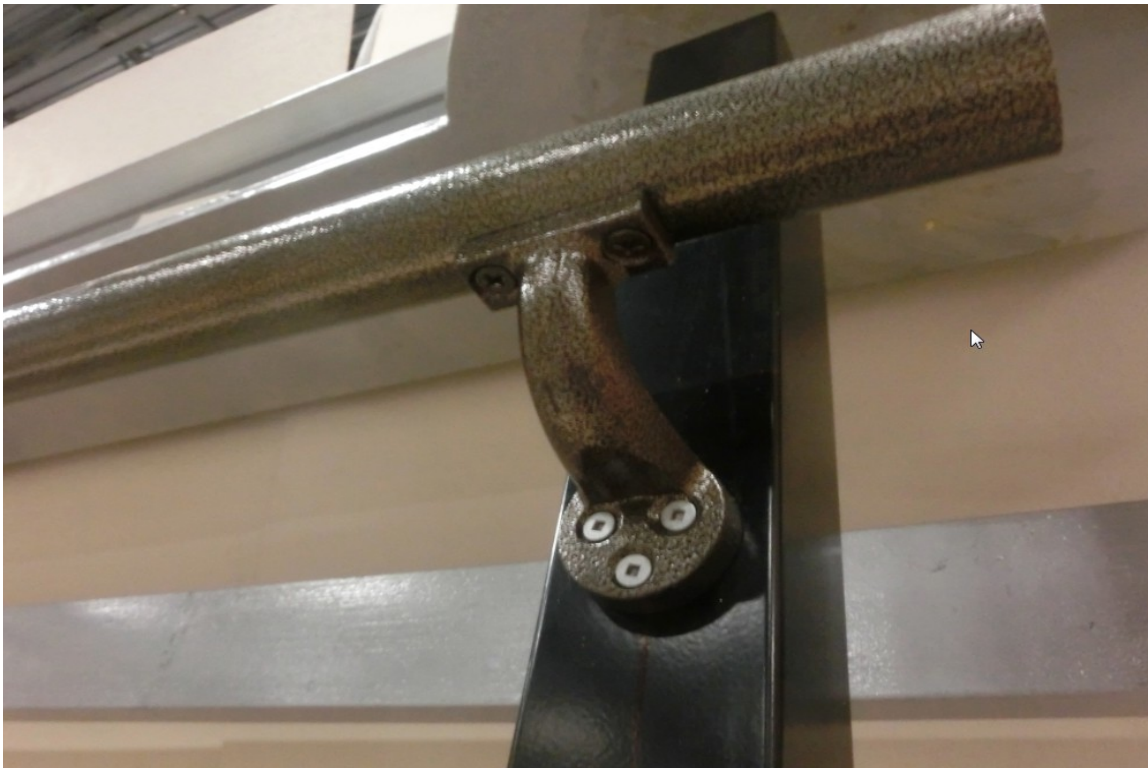
Photo 4: Typical Hand Rail Mounting
