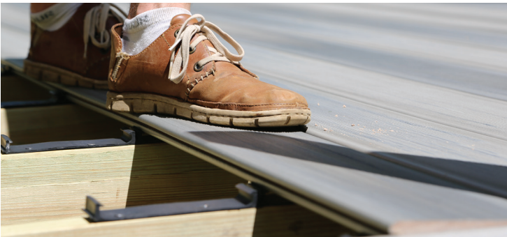
Position boards along each row of clips and step down or use a mallet on the board at each joist location to secure it into place.
