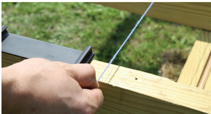
Snap a chalk line across the deck joists at a mark measured 21 5/8" (549 mm) (for 1" board overhang) from the outer edge or rim joist.
