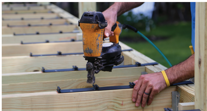
Position the end of each clip strip at chalk line and nail strips to each joist with side tabs tight against the same side of the joist.
